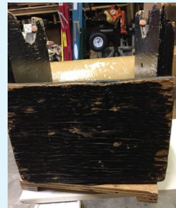
10. The front of the base had more delamination of the plywood layers, which led to splintering.
