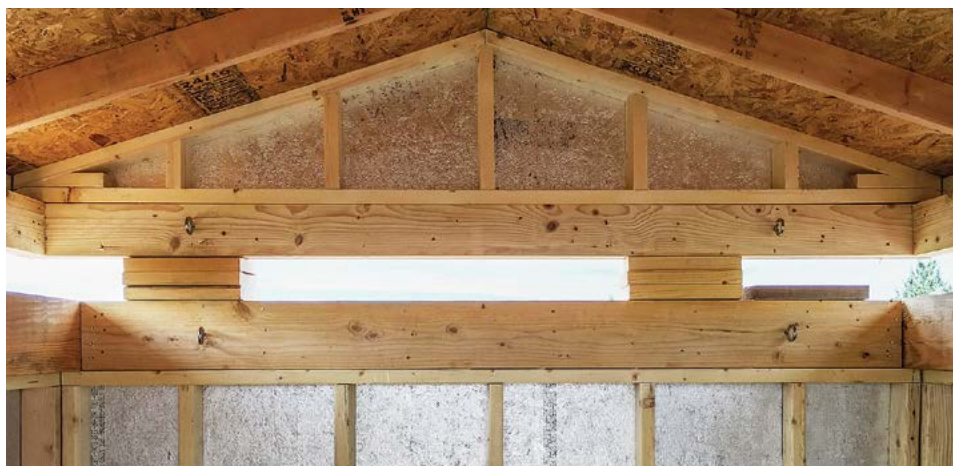
After toe-nailing was removed, the roof was temporarily supported on 2x6 stacks.
